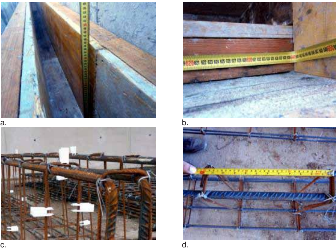
Figure 1. Verification of the dimensions and geometry of the mould (a. and b.), spacers employed to guarantee the concrete cover (c.) and verification of the positioning of the reinforcing bars (d.).
